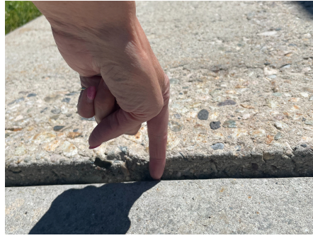
Example of a pathway with abrupt edges over 1/2 inch due to lifted concrete sections.
